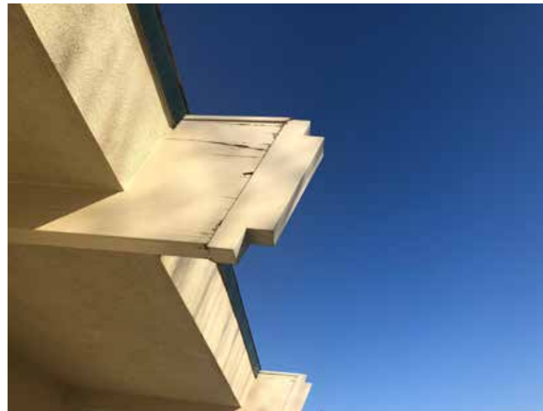
Glue-lam water damage
