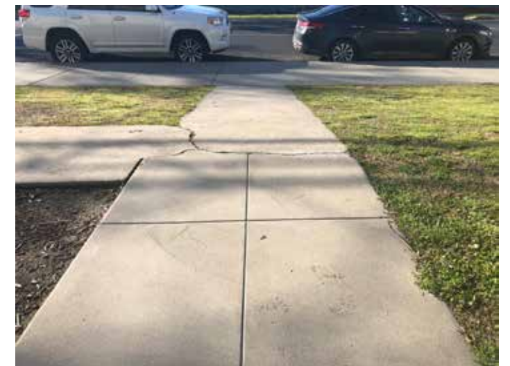
Non-compliant ADA path of travel
