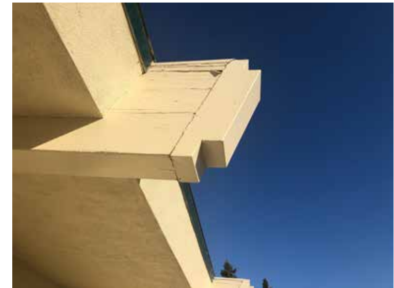
Glue-lam water damage
