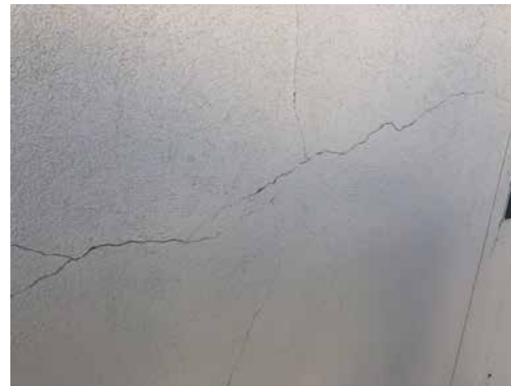
Exterior wall stucco cracks
