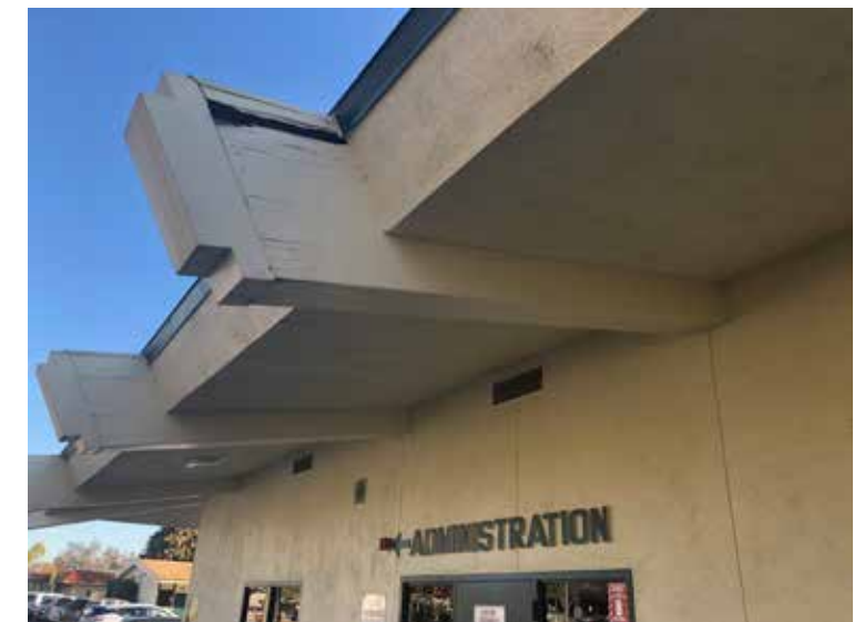
Glue-lam water damage
