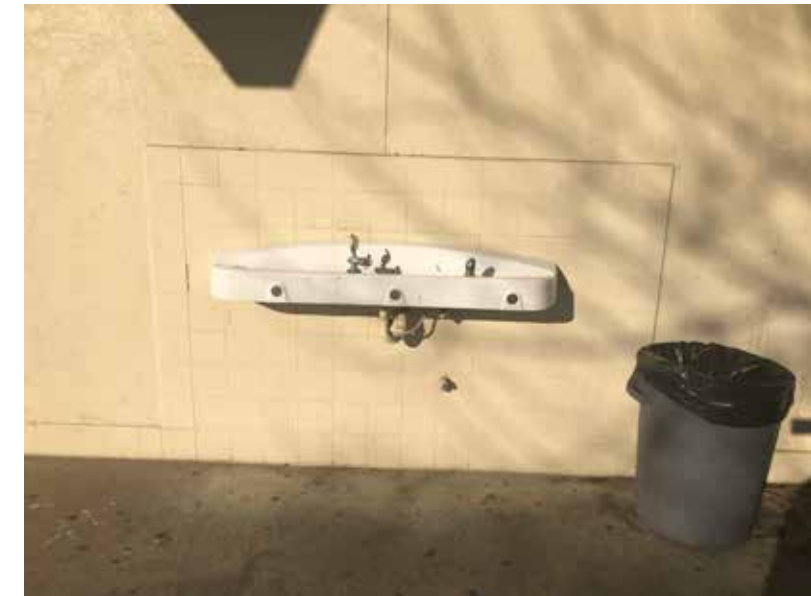
Building 10 drinking fountain
