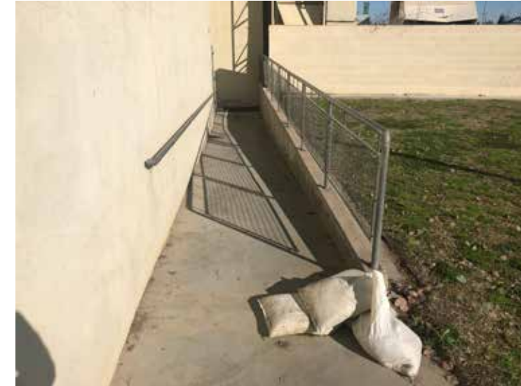
ADA access ramp flooding
