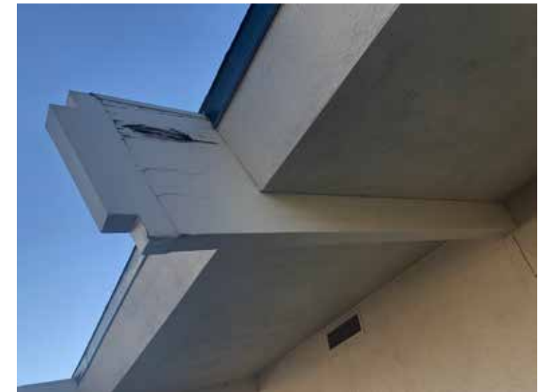
Glue-lam water damage
