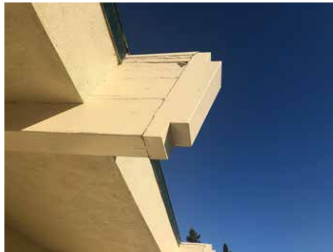
Glue-lam water damage
