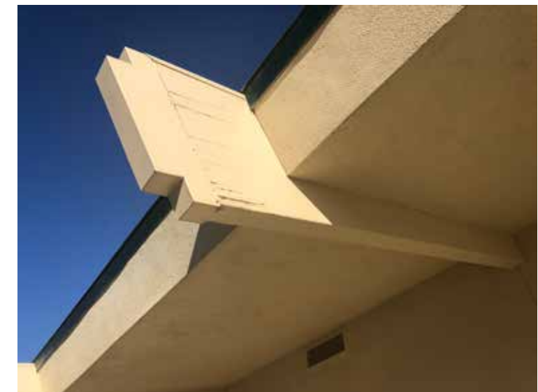
Glue-lam water damage
