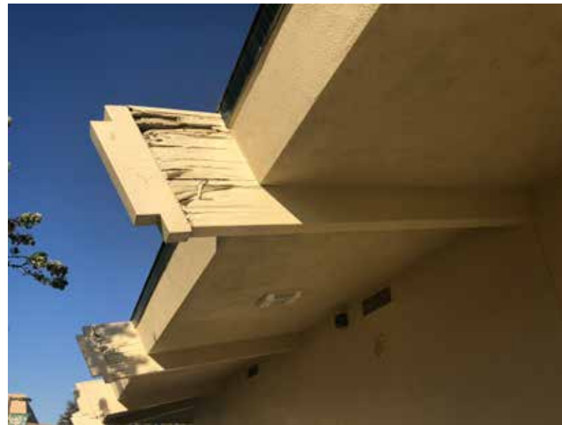
Glue-lam water damage
