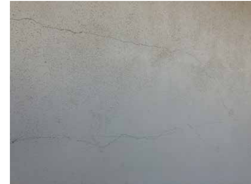
Exterior wall stucco cracks
